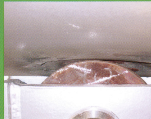
Pipe dent caused by a steel roller
